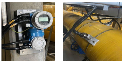
Figure 7: The Clamp-On Flow Meter in position at filter 5 outlet on site.
