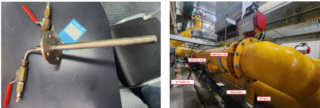
Figure 1 Existing Pitot Tube removed from pipework and the challenges of the GRP pipework
