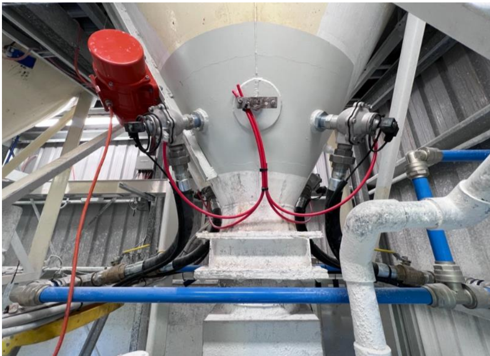
Figure 1 Vibrator and AirSweep® system installed on Lime Hopper 2
