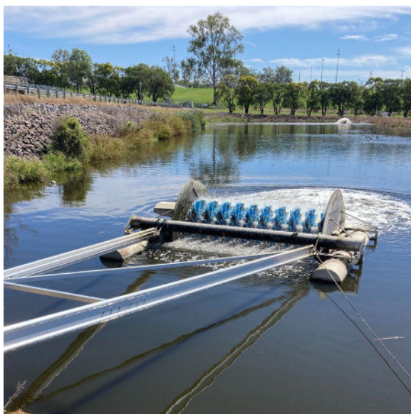
Figure 2 — Close-up of aerator in lagoon
