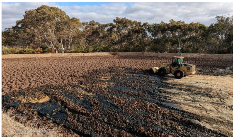
Figure 4: Attempted desludging of Lagoon 1 with wet sludge at Barossa WTP
