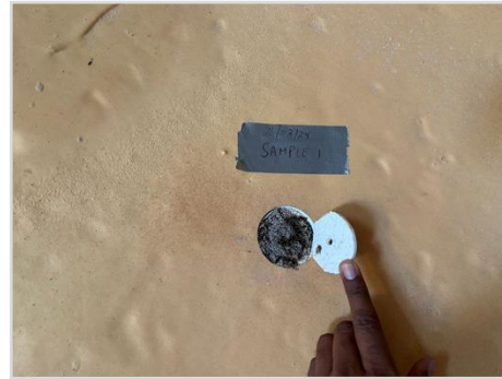
Fig. 3: A liner sample removed for testing.
