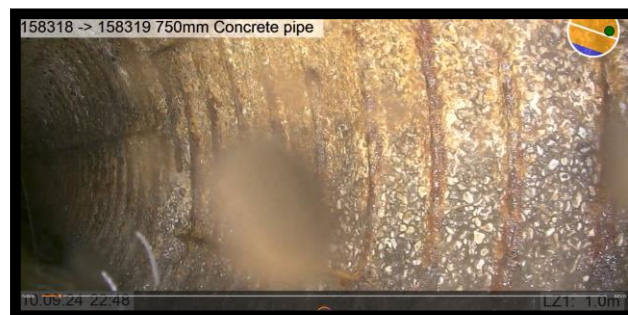
Figure 1: Evidence of concrete degradation in a section of main
