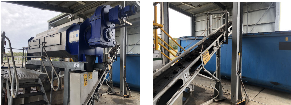
Figure 1 – Pulgul STP Existing Screw Press and sludge Conveyor
