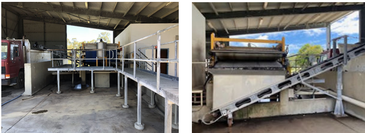
Figure 2 – Eli Creek STP Existing Belt Filter Press and sludge Conveyor
