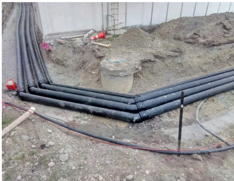
Christchurch Wastewater Treatment Plant. Courtesy Fusion Solutions
