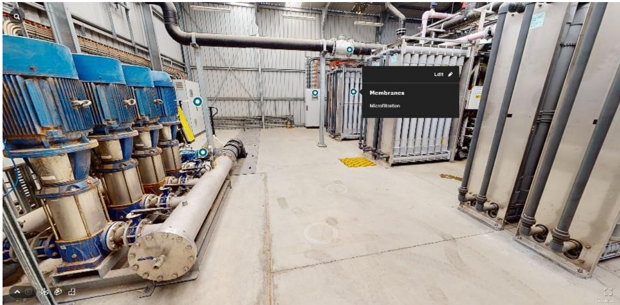
Figure 3: A Matterport scan of a Waste Water Treatment Plant with identified Points of Interest
