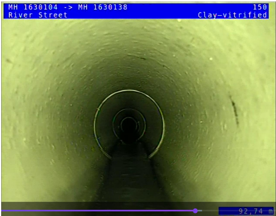
Figure 5: Example of CCTV Footage showing "Proof of clean" on asset
