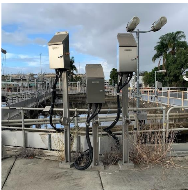
Figure 2: Example of the wind-up control panels installed after the 2011 flood
