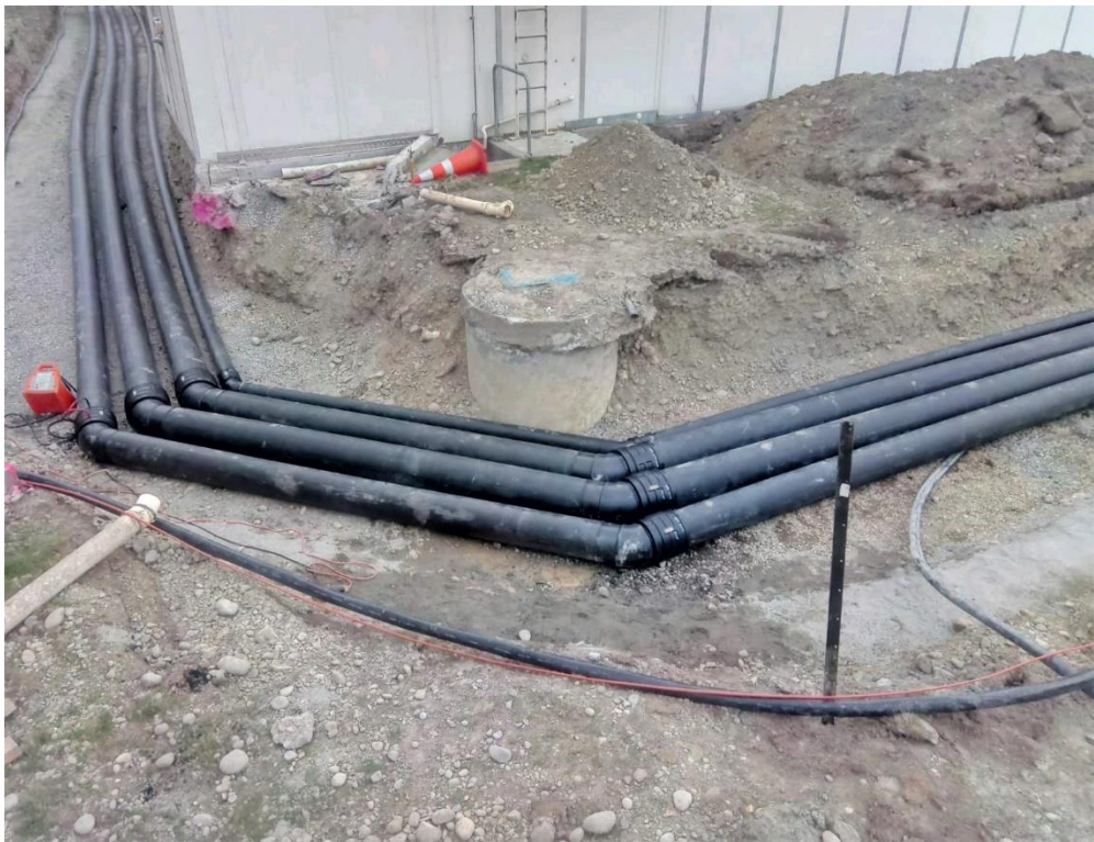
Christchurch Wastewater Treatment Plant. Courtesy Fusion Solutions
