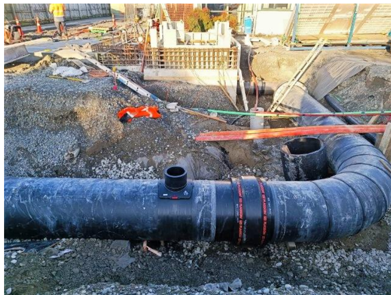
Christchurch Wastewater Treatment Plant. Courtesy Fusion Solutions.
