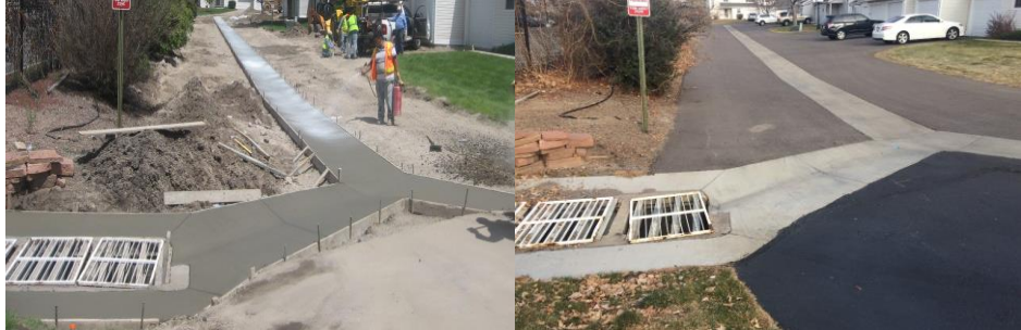
Figure 6: Concrete Company X Project – Town home Drainage System May 2015 (Left), December 2017 (Right)
