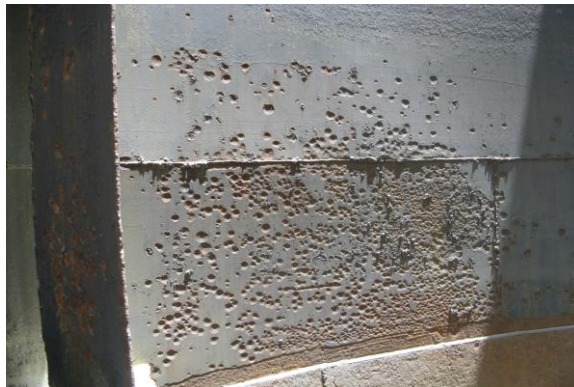
Figure 2.1 - Pitting corrosion occurring on thickener tank under a biofilm layer
