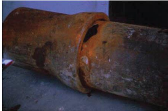
Fig 2.2 - Graphitic Corrosion on Bell and Spigot Ductile Iron Piping
