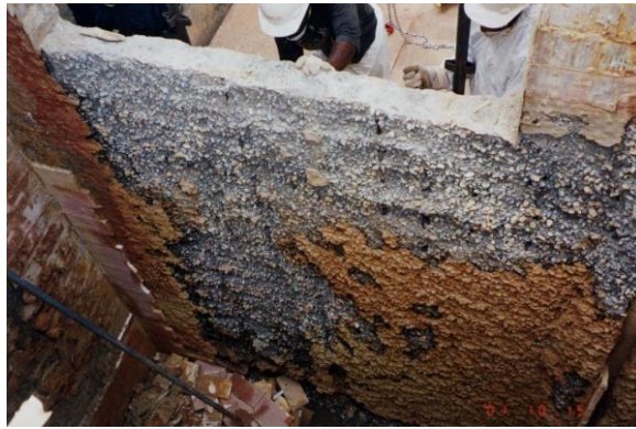
Fig 2.5 – Biogenic corrosion in enclosed head space of concrete bar screen chamber
