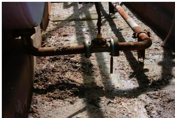
Fig 2.6 – Acid attack of concrete in sulfuric acid containment
