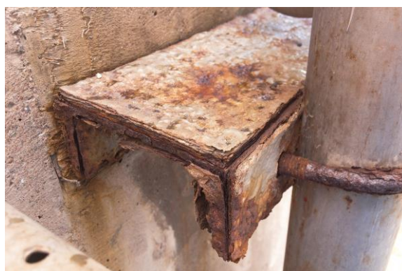
Fig 2.4 – Biogenic corrosion of pipe brace/support in wet well
