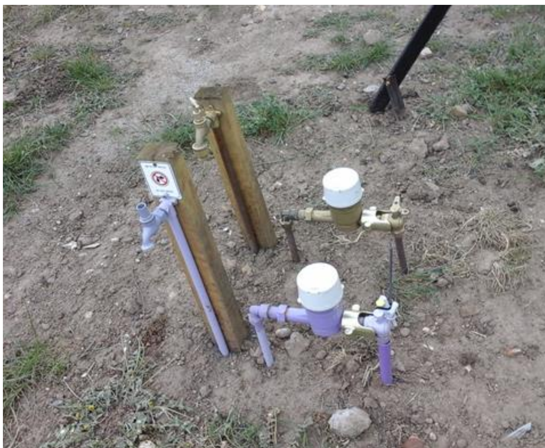
Figure 1 RW meter set up which is inspected at the R1 Inspection stage. The RW meter is on the left coloured purple.
