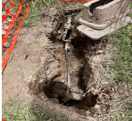
Figure 1 – Identified repeated leaking water service
