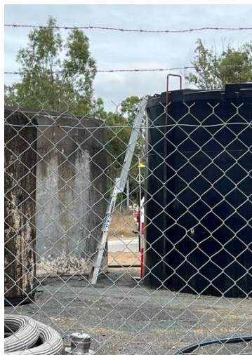
Figure 7: temporary tank connections
