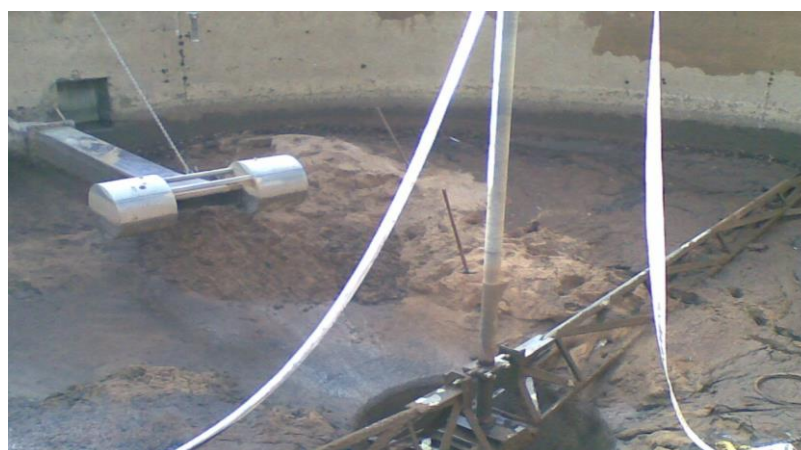
Figure 4: Sand build up in washwater recovery tank 1
