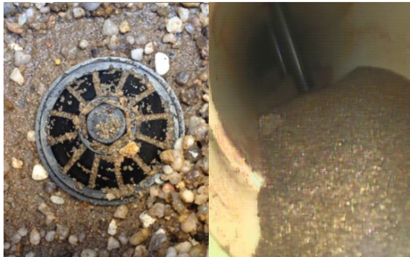
Figure 6: Blocked filter nozzle and sand build up in lateral pipework
