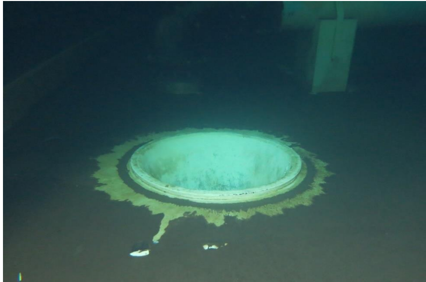
Figure 5: Outlet pipework flush with the floor and drawing in sediments
