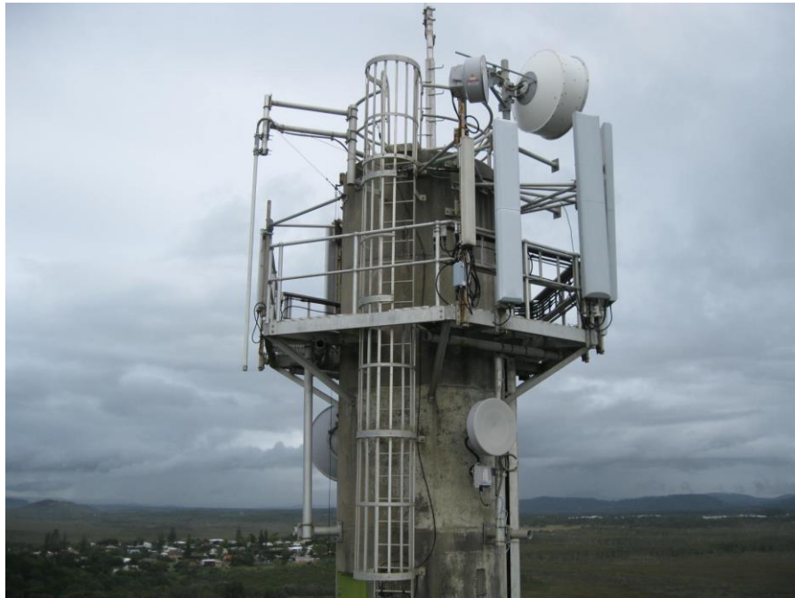
Figure 7: Telecommunication equipment restricts access to tank for maintenance
