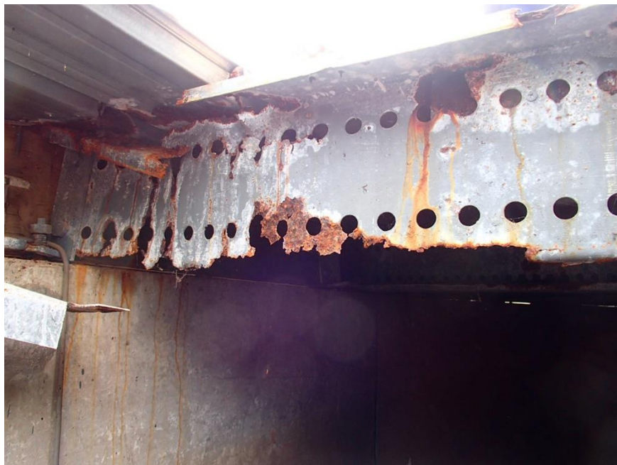
Figure 2: Zinc purlin corrosion due to a moist, chlorinated environment
