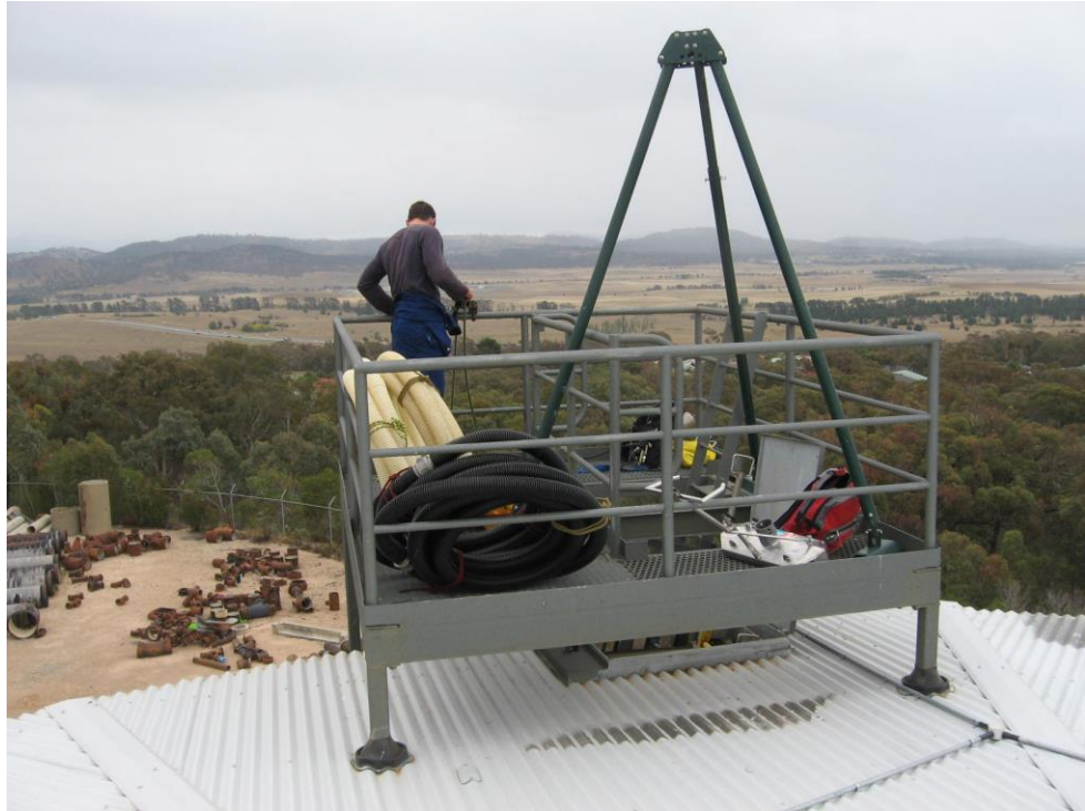
Figure 3: Platform design that restricts the safe working area and access into and out of the tank
