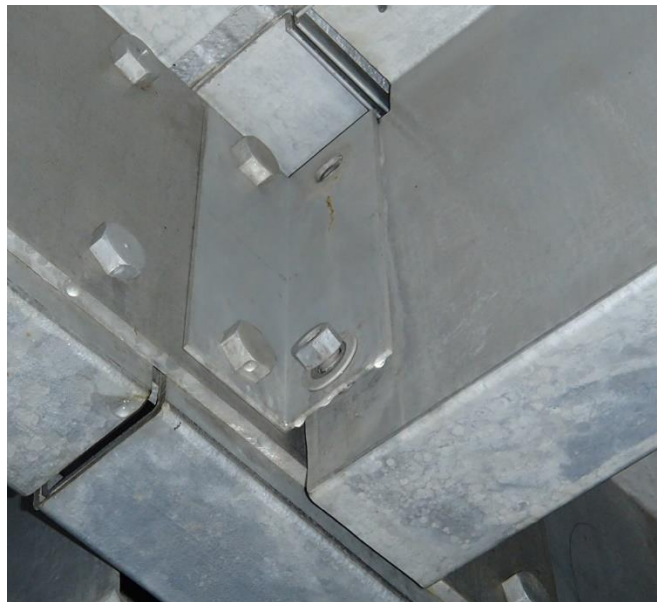
Figure 4: Aluminium roof framing bolts missing
