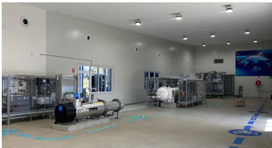
Figure 1: Quakers Hill PRW Discovery Centre Treatment Room with the Ultrafiltration, Reverse Osmosis, and UV-Advanced Oxidation Units and their Sample Panels.
