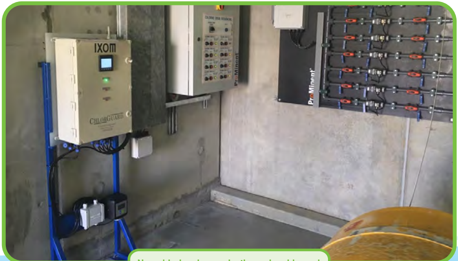
New chlorine drum selection solenoid panel.
