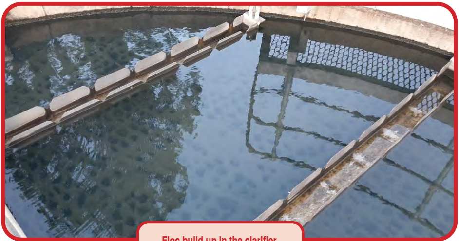
Floc build up in the clarifier.
