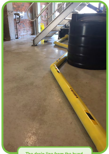
The drain line from the bund.
