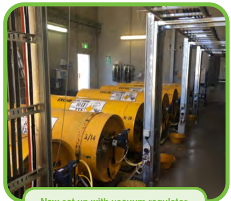
New set up with vacuum regulator connected directly to chlorine drum.
