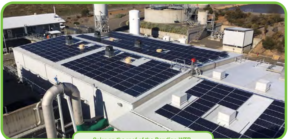
Solar on the roof of the Bendigo WTP.
