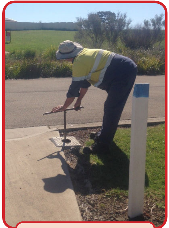
Opening an unlocked valve.
