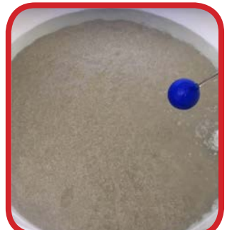
Final cleaned media added to the fluoride saturator ready for return to service.
