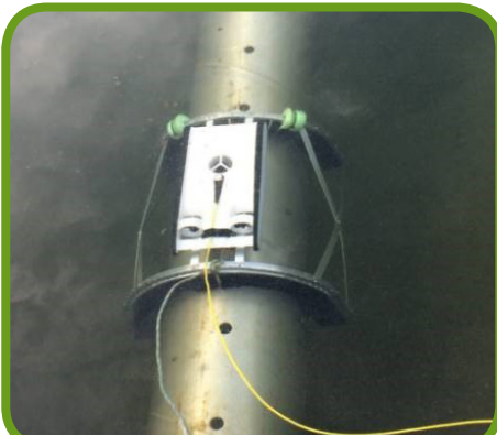
A fully cleaned launder.
