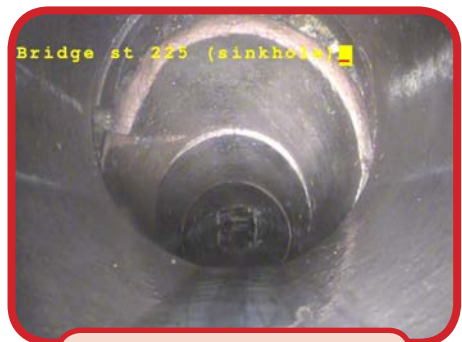
CCTV showing extent of the hole.
