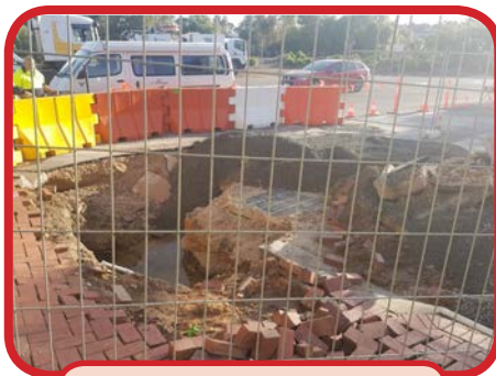
The sink hole at the surface.
