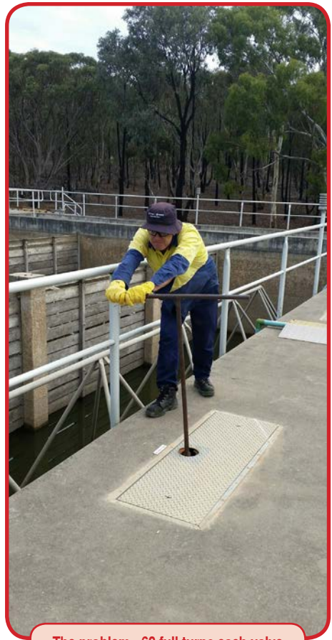
The problem - 60 full turns each valve
