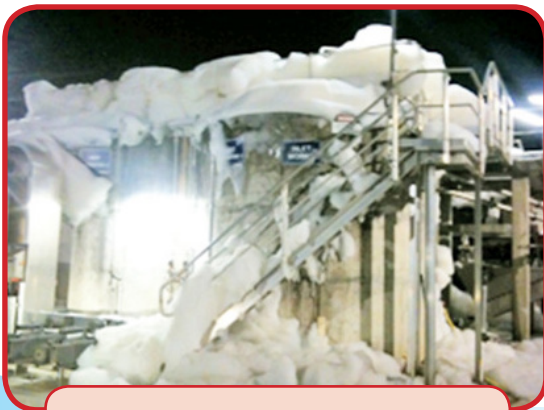
Trade waste shock causing foaming at Burpengary East STP
