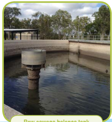
Raw sewage balance tank with wet weather bypass bellmouth
