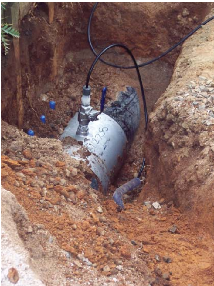
▼ The solution - new ph correction dosing point.
