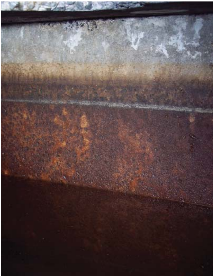
▼ The problem - staining of water storage tank walls.
