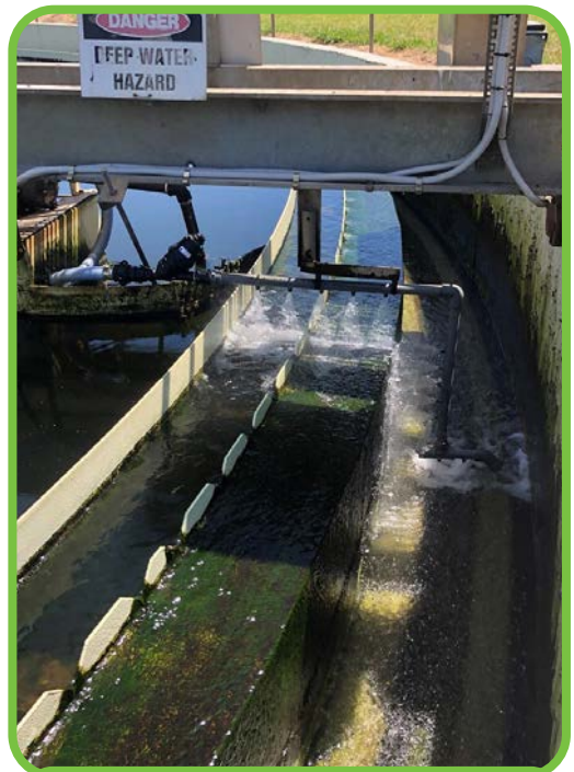
Spray system and clean clarifier outlet channel
