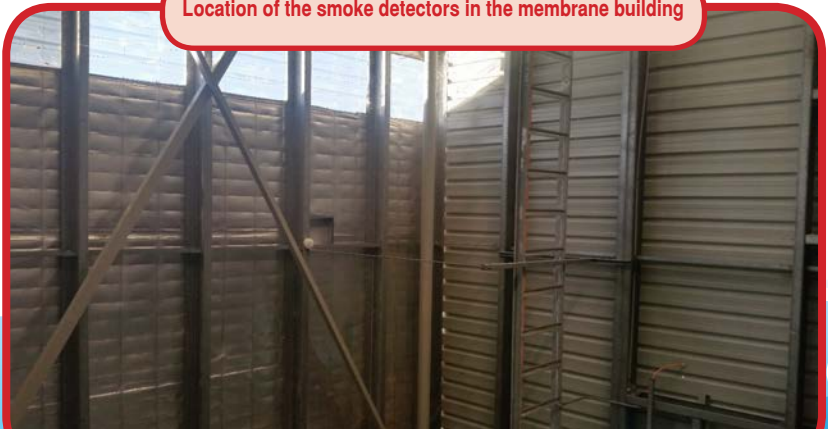
Location of the smoke detectors in the membrane building
