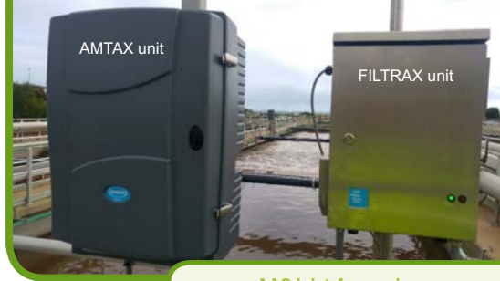
AAC Inlet Ammonia Analyser Installation
