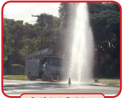
Burst Spring-top Fire Hydrant. Example of an incident causing water outages
