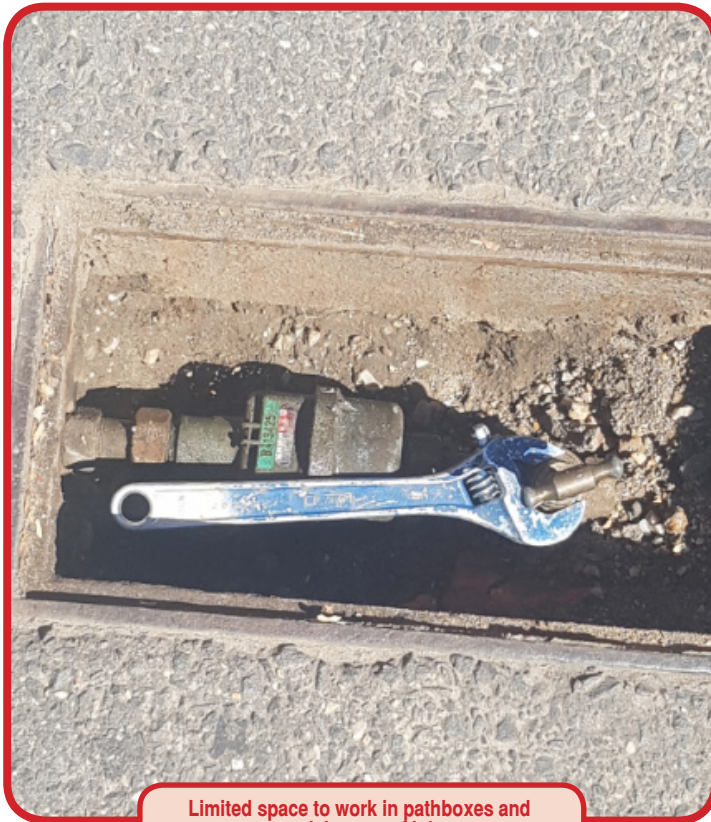
Limited space to work in pathboxes and potential cause of injury.
