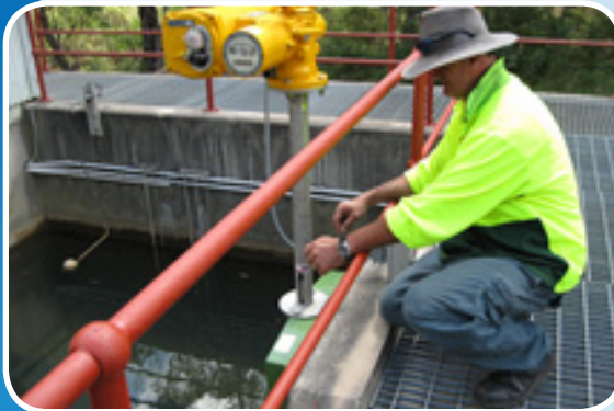
The original working position for the actuators
