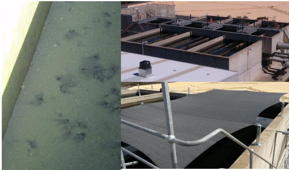
Figure 1: Bendigo WTP BACs - (L) 2011 bog ore prior to covers, (Top R) 2012 before covers, (Bottom R) 2016 during cover installation
