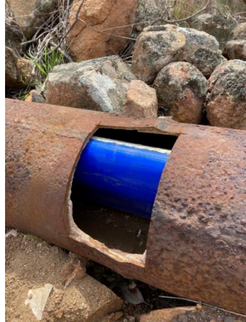
Figure 5: DN200 Primus Line installed inside host pipe (DN250 MSCL) ready for pressure testing
