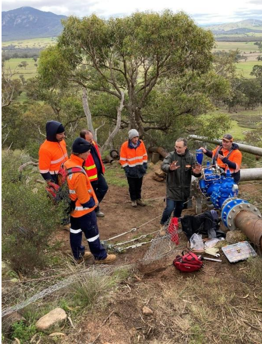
Figure 6: Combined Pipeline Commissioning and Operator Training. Photo of Pressure Sustaining Valve site - located at the downstream end of the relined section. (CH 1,400m)
