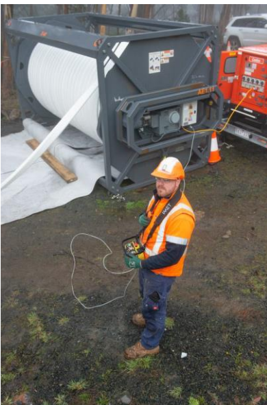
Figure 3: Unwinding DN200 Primus Liner from Transport Drum at Upstream End (Length: 1.4km)
