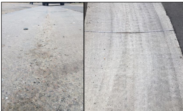
Figure 7: Concrete Company C Project – Town home Drainage (December 2017; 31-months old); Reference (Left) and CNT Additive (Right)
