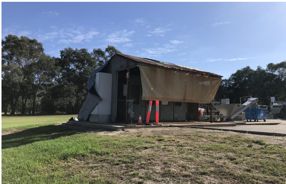
Image 1 - Existing installation with tarps to protect the weary switch board from the weather.
