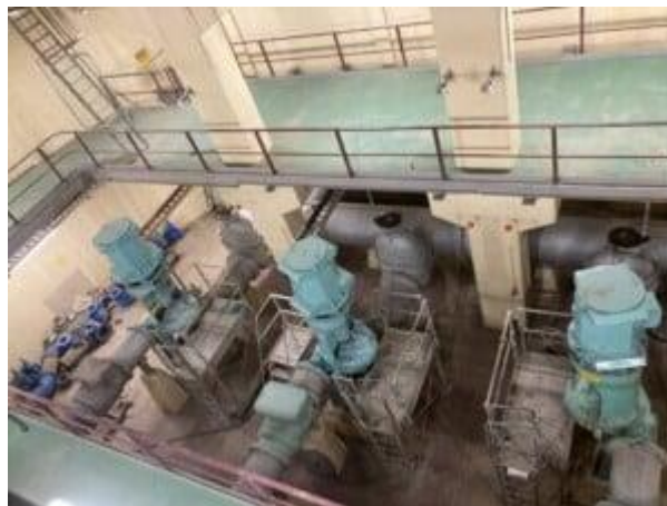
Figure 1: St Mary's Sewage Pump Station – Vertical split pump units, Chesterton 442 Split Seal and overhaul including ARC Industrial Coatings.
