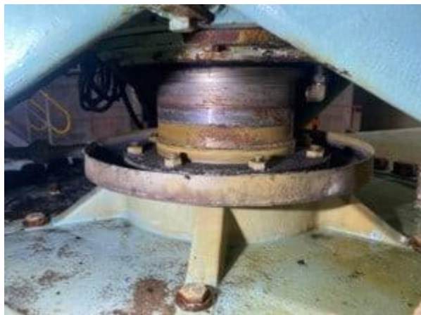
Figure 2: Main outfall pump packed gland upgrade to Chesterton 2211 DualPac®
