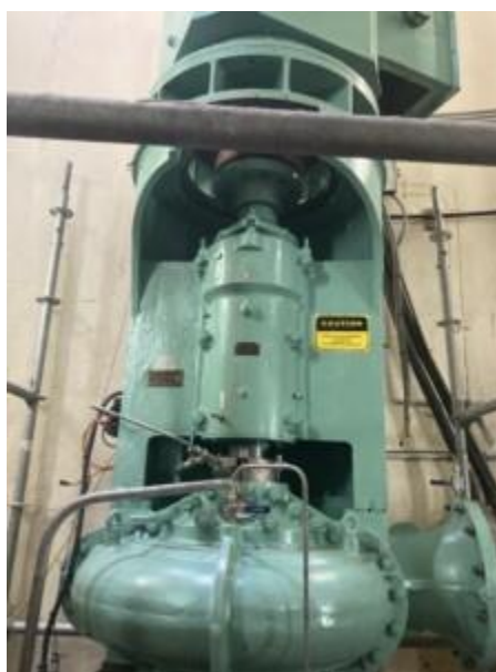
Figure 7: Vertical Sewage pump unit overhauled with hardened 420SS casing & impeller rings combined with ARC ceramic coating, reducing erosion wear.
