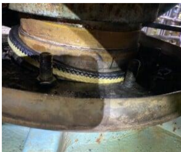
Figure 3: Outfall pump gland being re-packed with 1" square Chesterton 2211 DualPac®
