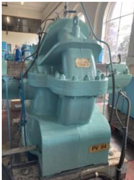
Figure 6: Potable Water pump overhauled with Chesterton ARC ceramic coating and 1810 cartridge seals
