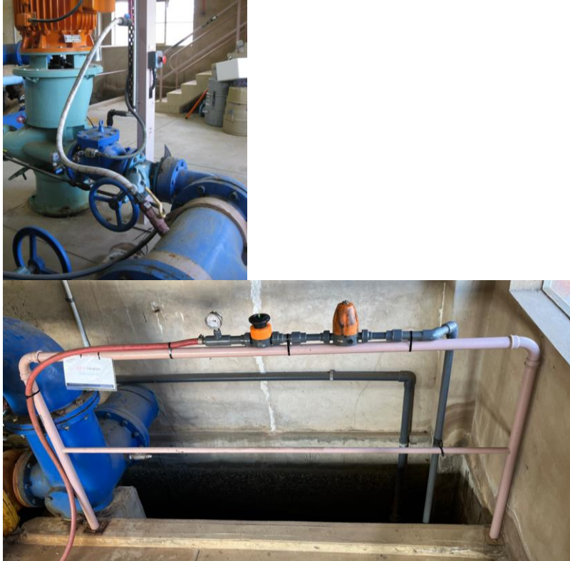
Figure 2: Old (left) and New (right) temporary fluoride dosing point
