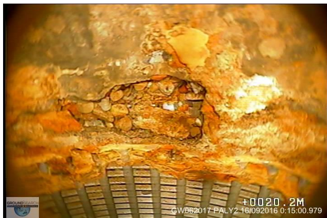
Figure 2 Corrosion at dissimilar metals mild steel casing and stainless steel screen welded.
