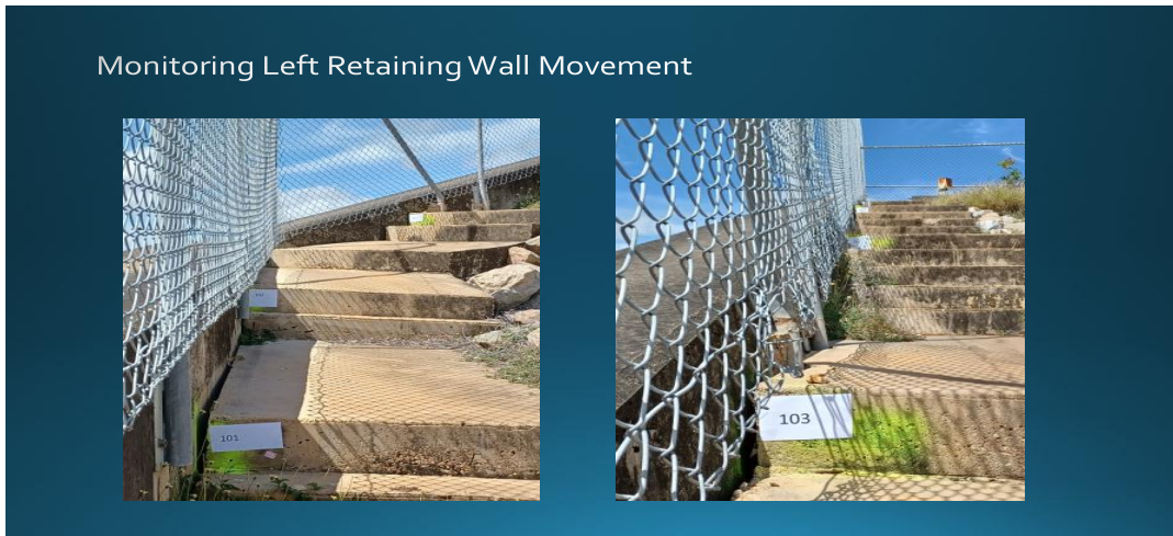
Figure 1: Gap between the Dam Left Retaining Wall and Staircase of Left Embankment
