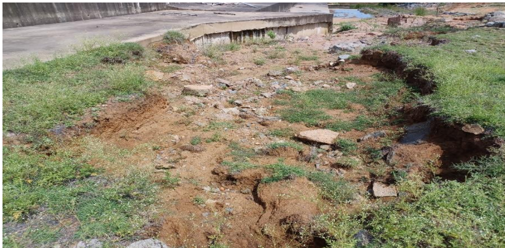
Figure 4 Gully area below the right concrete terrace of the dam being monitored.
