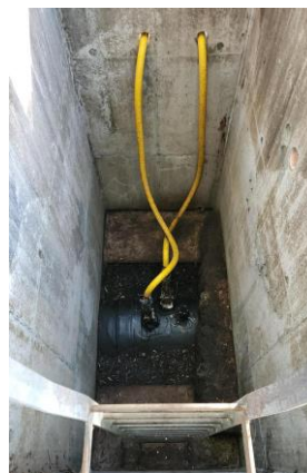
Figure 2 Pre lime dosing pit
