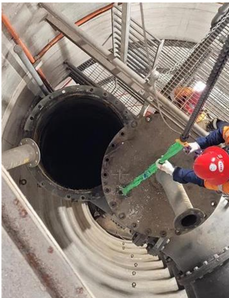
Figure 5 Blanking plate at intake tower
