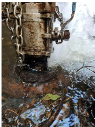
Figure 1 Leak at injection point
