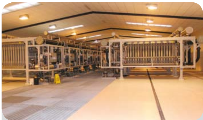
The Oropi WTP and there is tons of room to add more membranes in future.
