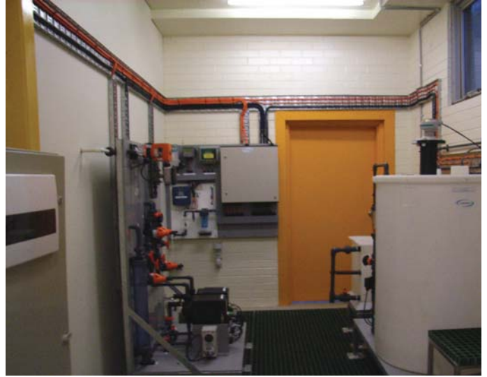
Morwell Water Treatment Plant Fluoride Room
