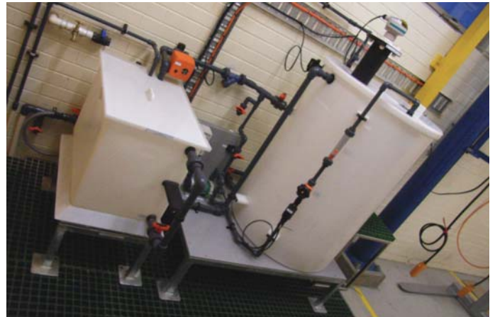
Saturation and Dosing Tanks
