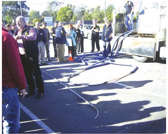
The 'us' - Utility Services pipe relining system in action at the distribution seminar
