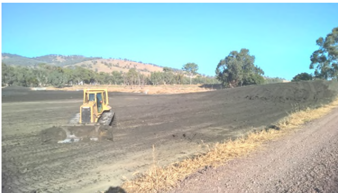
Figure 1: West Wodonga WWTP Drying Pans
