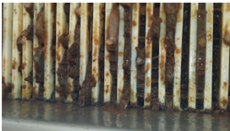
Figure 2: Sludged Membrane Cassettes
