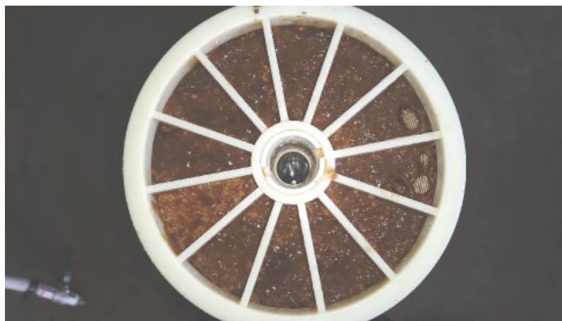
Figure 1: Solids Ingress into the RO
