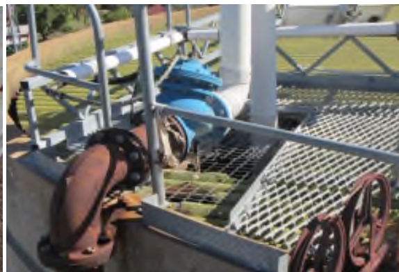
Figure 4: Open Roof Areas Allowing Drainage and Vermin Entry
