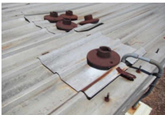
Figure 3: Unsecured Entry Hatch
