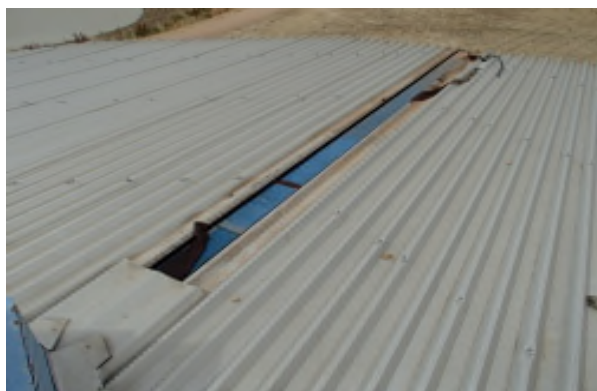
Figure 1: Roof Ridge Cap Missing
