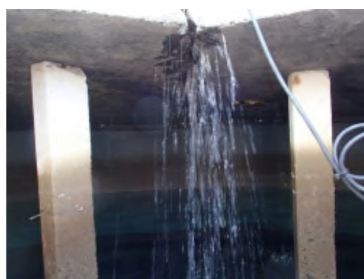
Figure 6: Internal Evidence of BoW Test Failure
