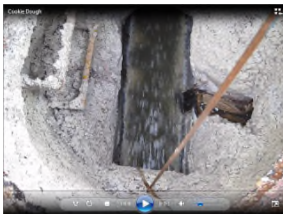
Figure 1: Sewer Manhole Concrete Corrosion
