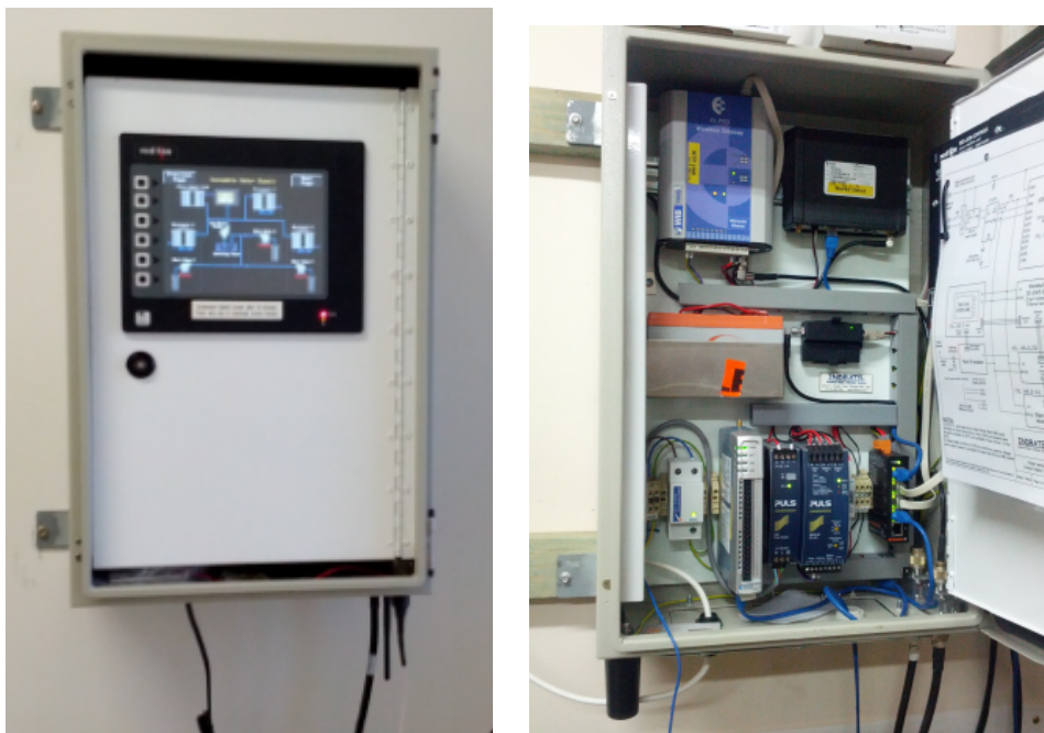
Figure 3: Cobar Shire HMI & Radio Cabinet
