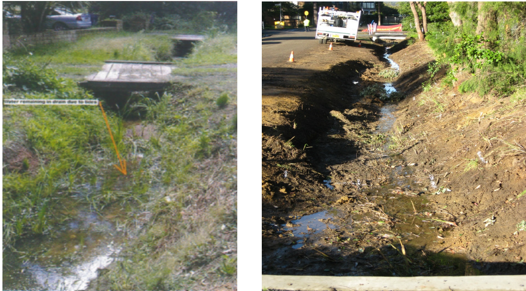
Figure 5: The Existing Drainage Problem
