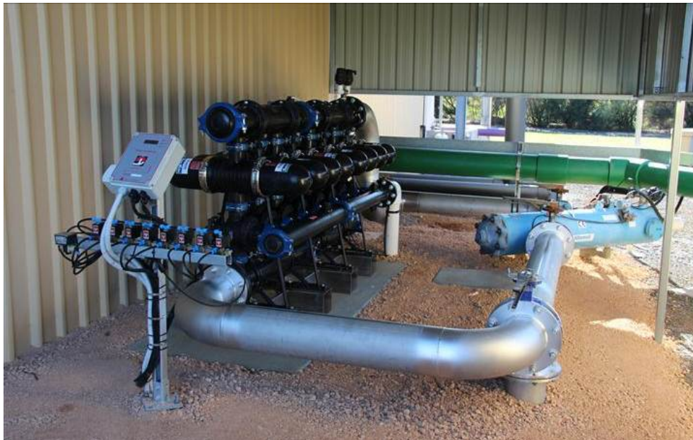
Figure 4: Pre-filtration system post upgrades
