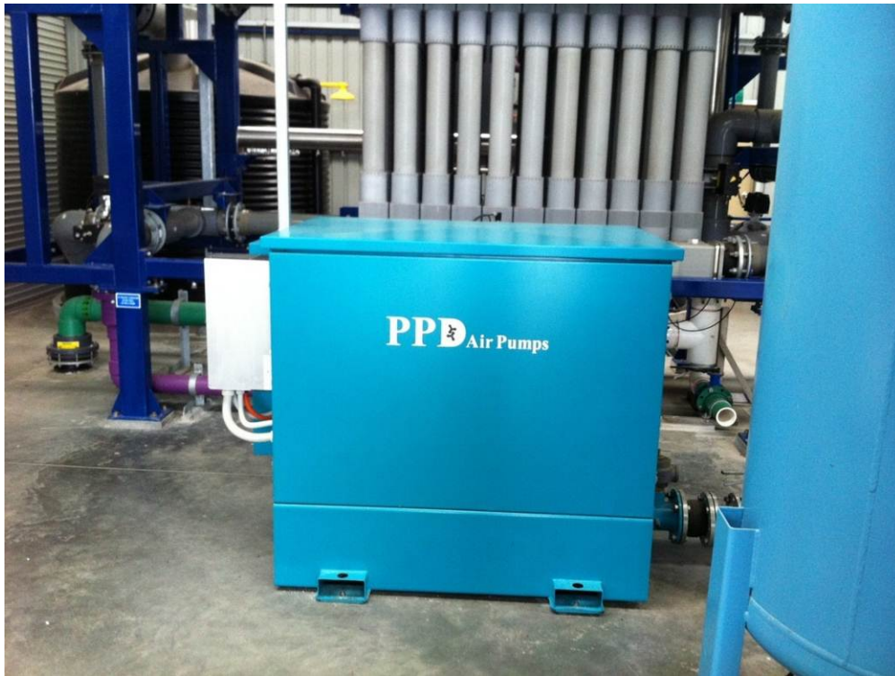
Figure 8: Blower installed at Willaura Membrane Filtration Unit for low pressure backwash
