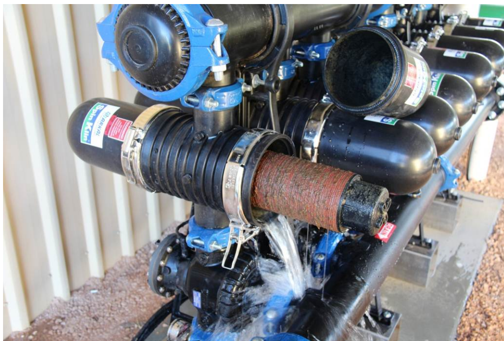
Figure 5: Disc filters doing their job before backwash
