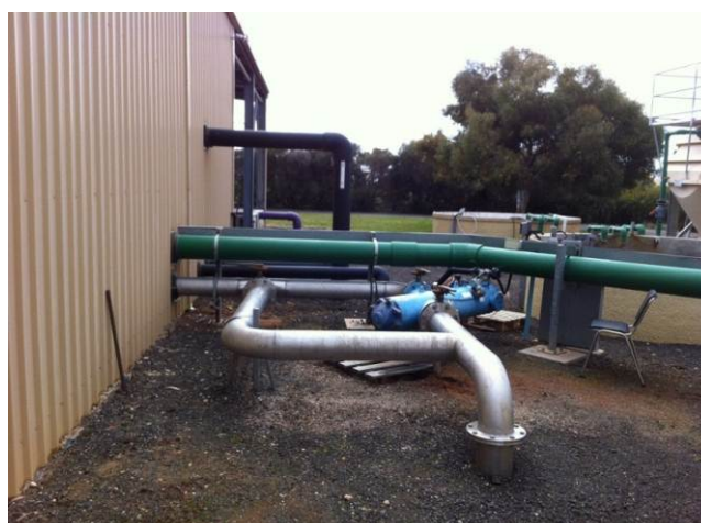
Figure 3: Pre-filtration system prior to upgrades between storages and water treatment plant
