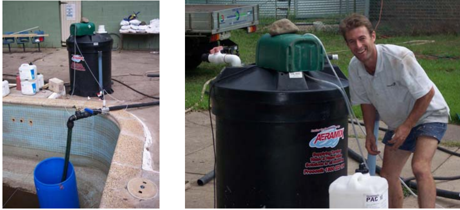
Figure 9: PAC mixing system and Jerry rigged rapid mixing and diffuser tank
